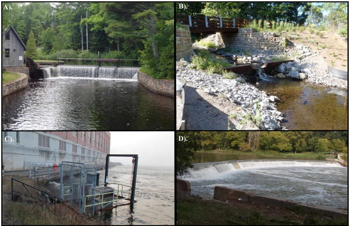
Figure 2-1. Examples of existing structures that are lowermost barriers to sea lamprey passage: (A) Rock River Dam, MI (Lake Superior); (B) Wheelway culvert barrier on Tannery Creek, MI (Lake Michigan); (C) Alexander Generating Station on the Nipigon River, ON (Lake Superior); and (D) Humber River Dam, ON (Lake Ontario). Photos courtesy of the U.S. Fish and Wildlife Service and Fisheries and Oceans Canada.
