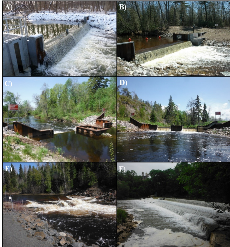
Figure 3-3. Examples of fixed-crest barriers: (A) purpose-built sheet pile barrier in Trail Creek, IN (Lake Michigan); (B) purpose-built sheet pile barrier at the Carp Lake outlet, MI (Lake Michigan); (C) upstream view and (D) downstream view of purpose-built sheet pile barrier in the Still River, ON (Lake Huron); (E) purpose-built concrete barrier with natural falls in the Wolf River, ON (Lake Superior); and (F) modified concrete Streetsville Dam in the Credit River, ON (Lake Ontario)(although repaired, sea lamprey have regularly escaped since 1980). Photos courtesy of the Great Lakes Fishery Commission and Fisheries and Oceans Canada.
